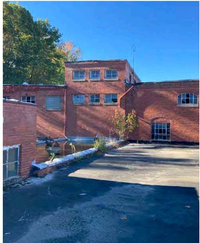
High bay pumping gallery clerestory windows adjacent to covered storage tank - foreground. East side of filtration gallery background.
